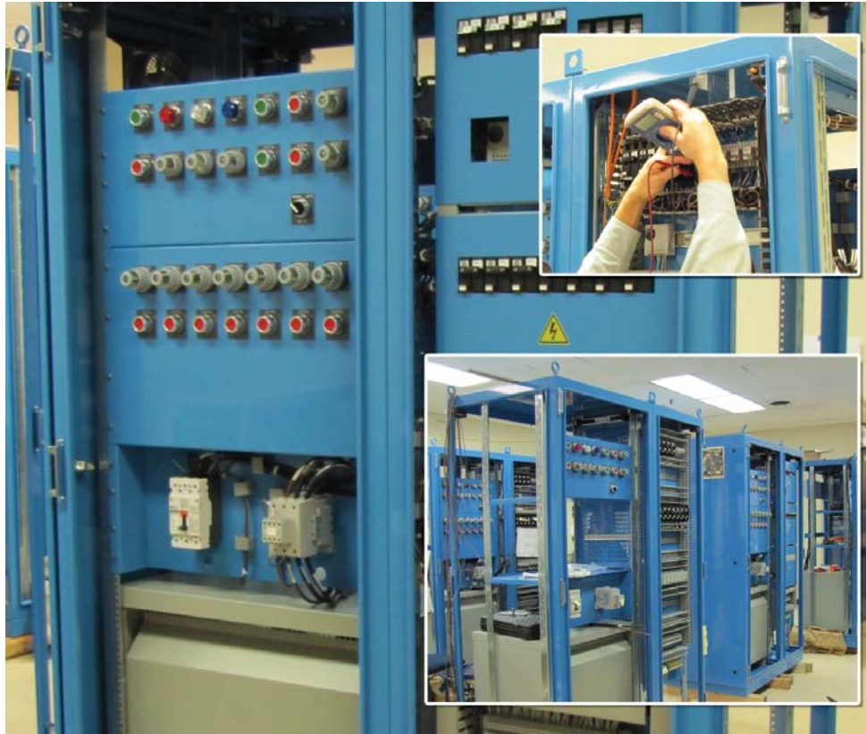
Electromechanical Services Room
